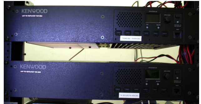
Kenwood UHF Repeaters (Link Radios)
