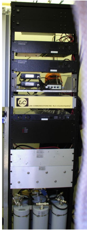
SDARC Bruin Repeater Rack
